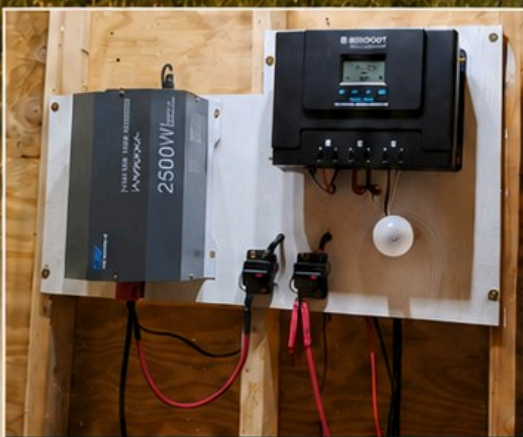
RELIABLE POWER SYSTEMS
